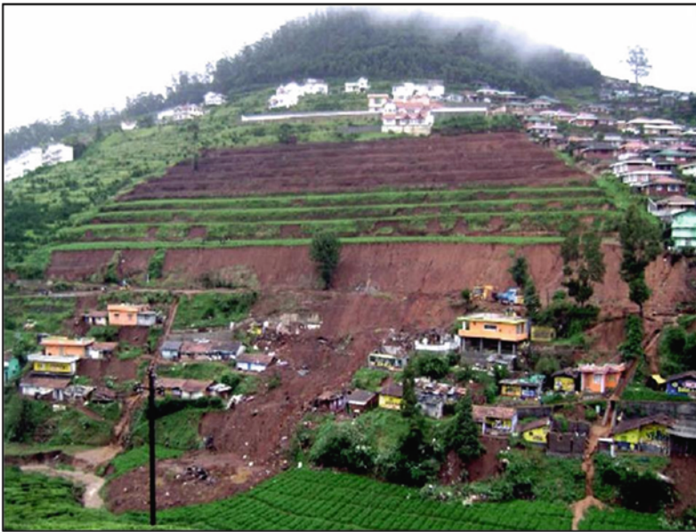
Fig. 3.52 A cutting in the residual soil slope at Ootacamund in State of Tamil Nadu India, as shown in the picture, failed because of the combined effect of progressive weakening with the passage of time, poor maintenance, and inadequacy of drainage in the rainy season
