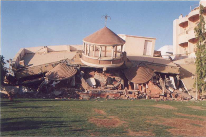
Fig. 3.16 A hotel in Gandhi Nagar collapsed during the Gujarat earthquake of 26 January 2001. This was entirely avoidable had the building design been faithful to the design codes for seismic zone V of the seismic zonation map of India
