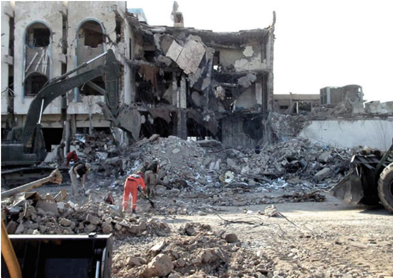
Fig. 5.4 The view of the U.N. building (popularly known as the Canal Hotel) after terrorist bombing on 19 August 2003
